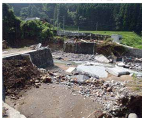
橋梁被災(流失)状況(小園橋)
